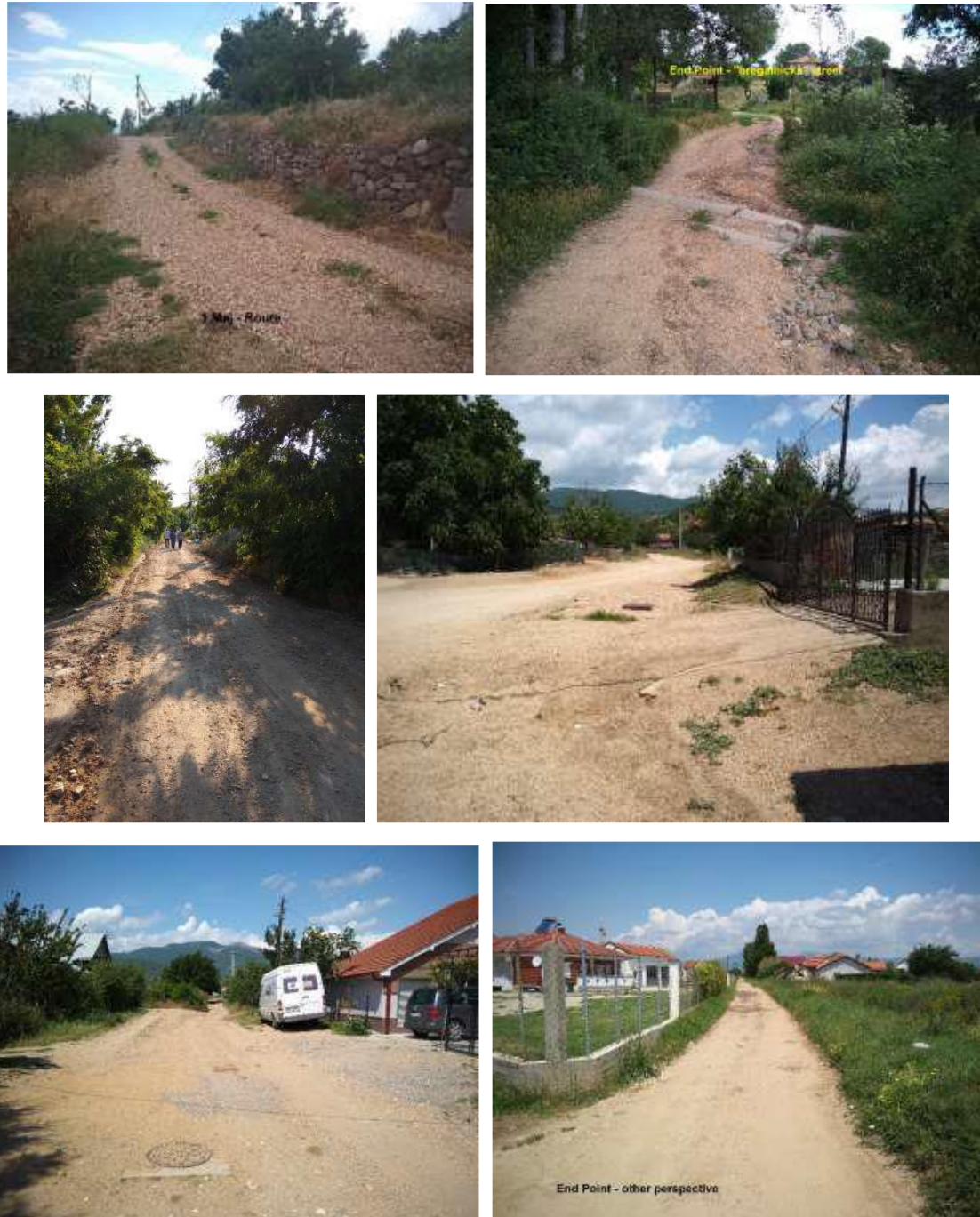
Figure 2 Condition of the existing local roads/streets that will be reconstructed/rehabilitated under the LRCP
